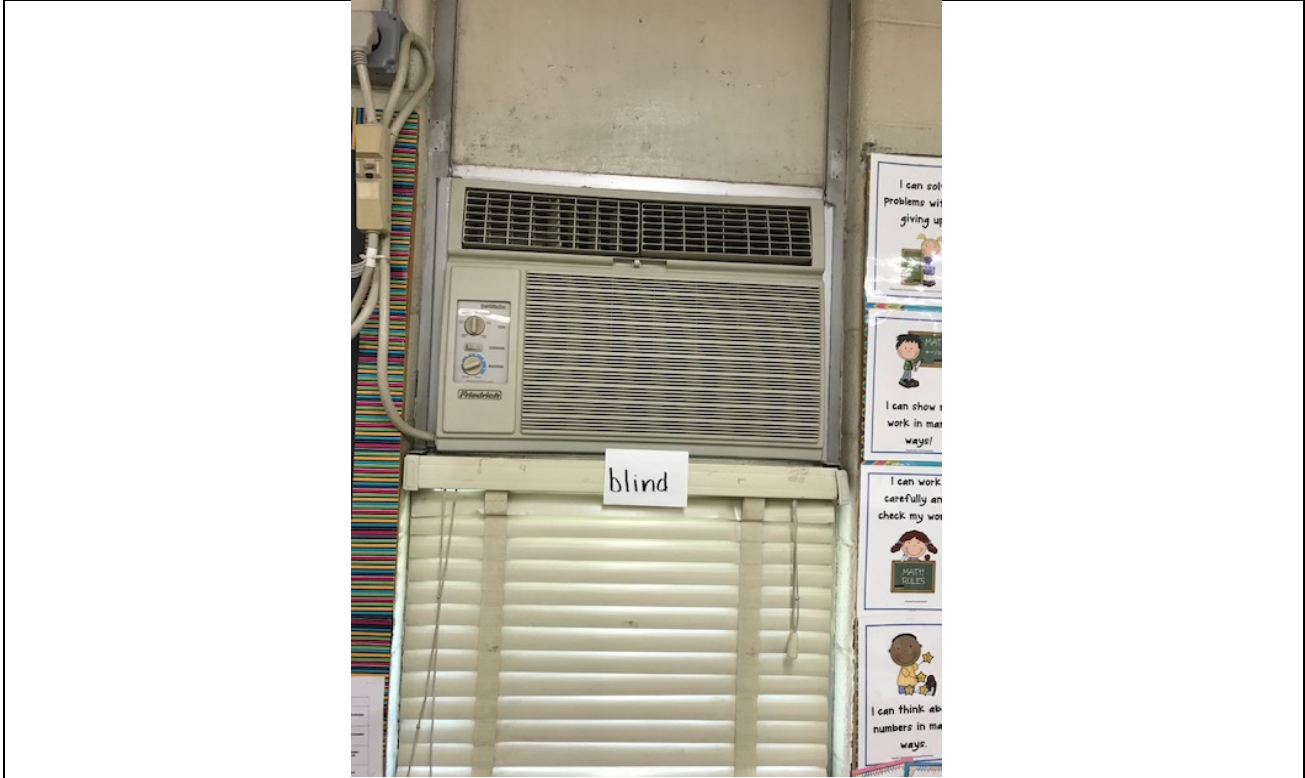
Photo 3: Classroom 20 – Window Mounted HVAC Unit with dusty grills
