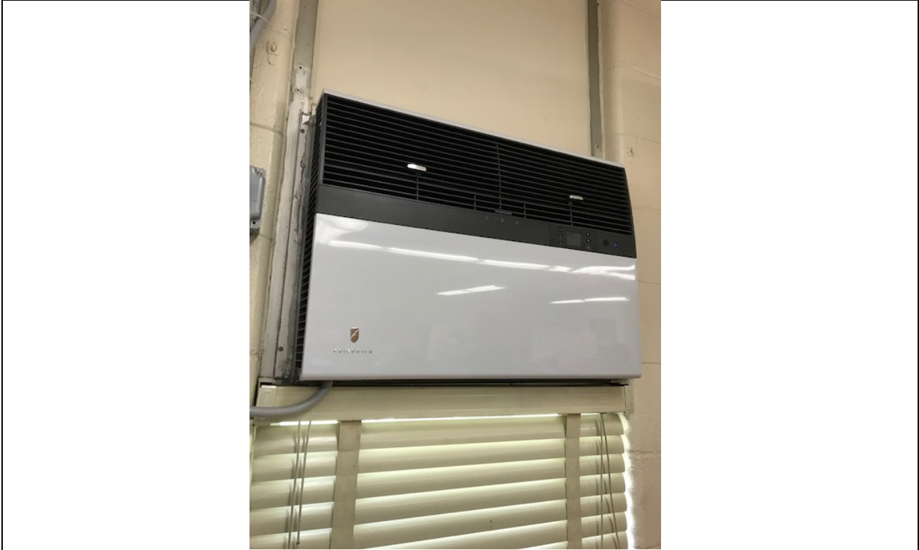
Photo 1: Classroom 15 – Window-mounted HVAC system operating.
