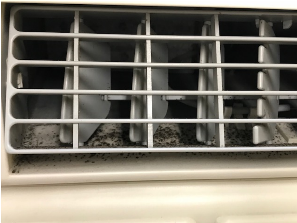
Photo 5: Classroom 10 – Window-mounted air conditioning unit with mold infested return grills
