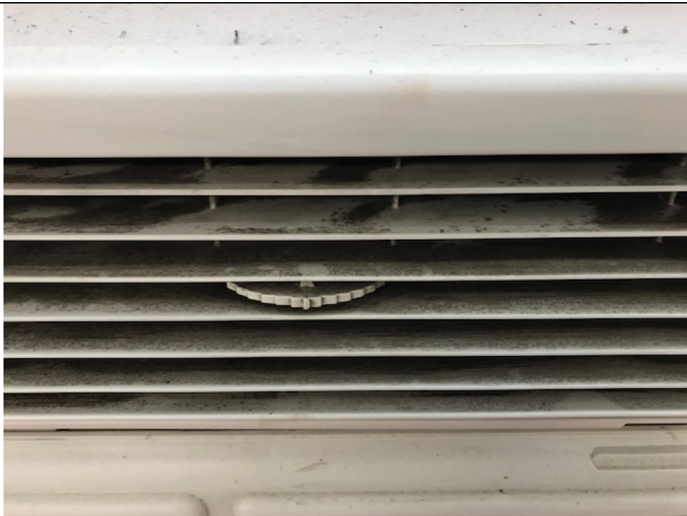
Photo 6: Library – Window-mounted air conditioning unit with mold infested return grills
