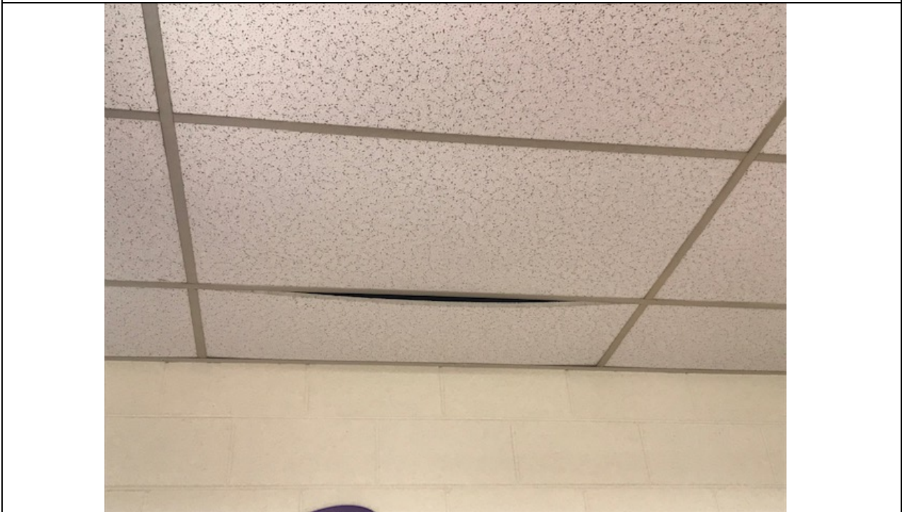
Photo 2: Classroom 15 – Protruding Ceiling Tile.
