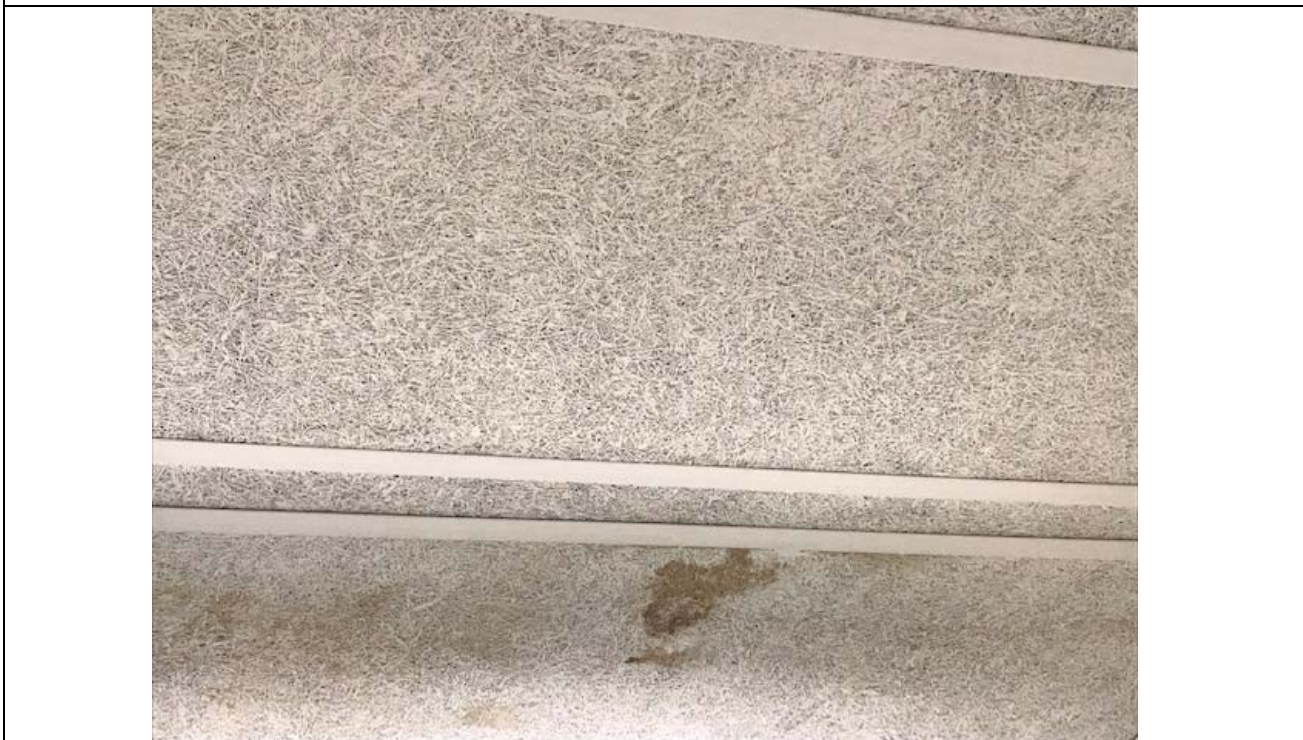
Photo 4: Classroom 101 – Water-stained ceiling tile.
