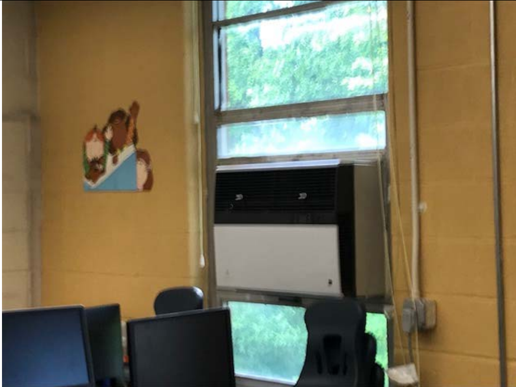
Photo 1: Library – Wall Mounted Air Conditioning Unit.
