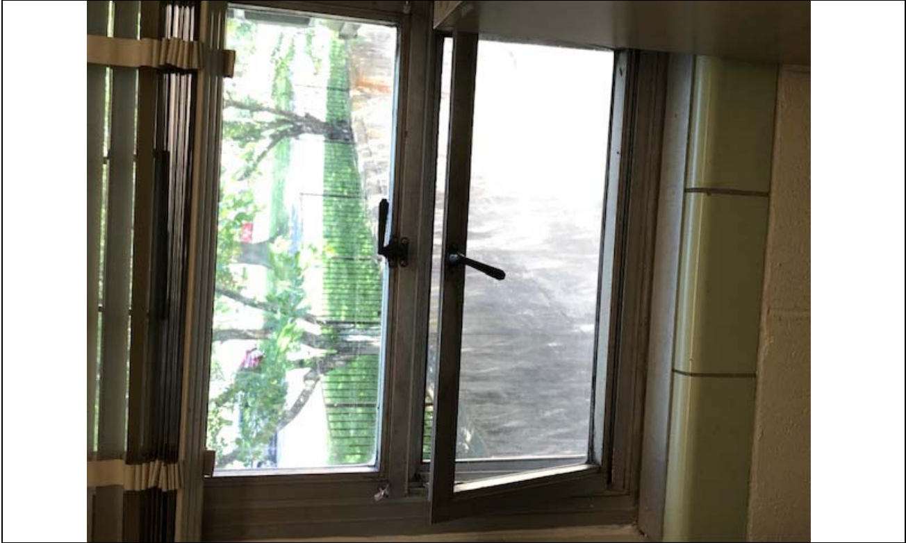
Photo 7: 1 st Floor Classroom 21 – Window left open.
