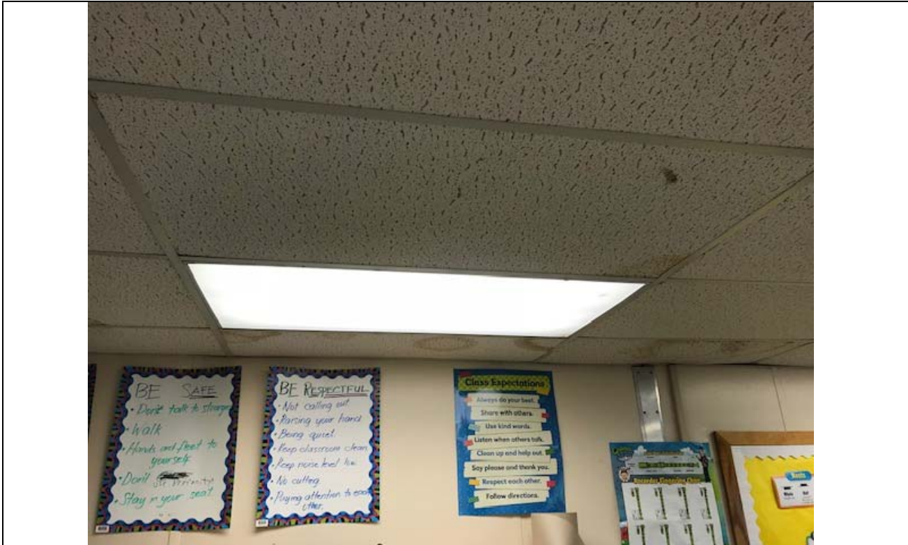
Photo 5: Temporary Building: Multiple water-stained ceiling tiles on ceiling.
