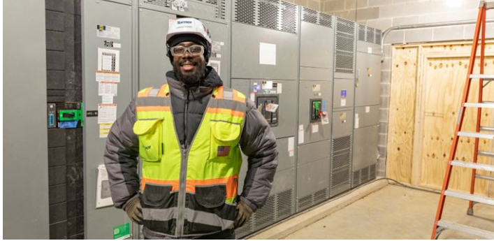
Electrical Switchgear Power Supply
