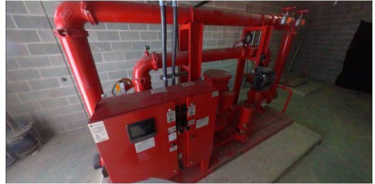
Sprinkler Pump Room
