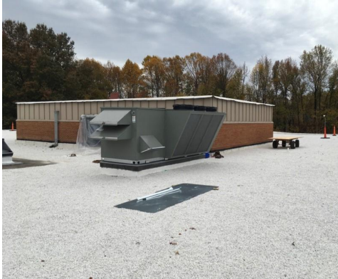
New, Packaged Rooftop Unit
