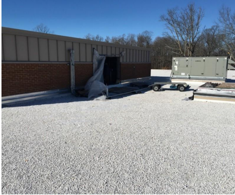
New, Packaged Rooftop Unit
