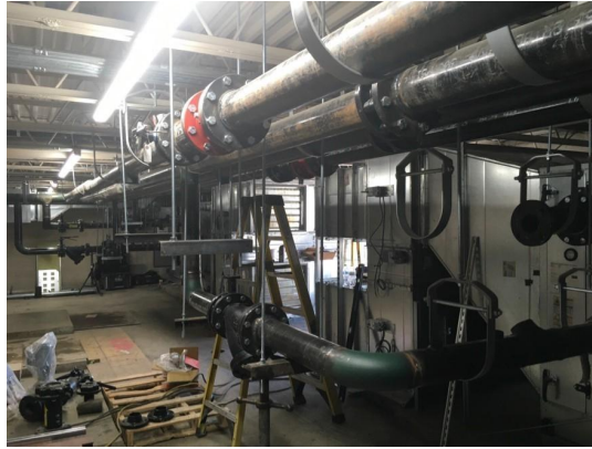
Hydronic Heating/Cooling Distribution Piping and Air Handling Units
