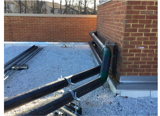
Roof Mounted Hydronic Cooling Distribution Piping
