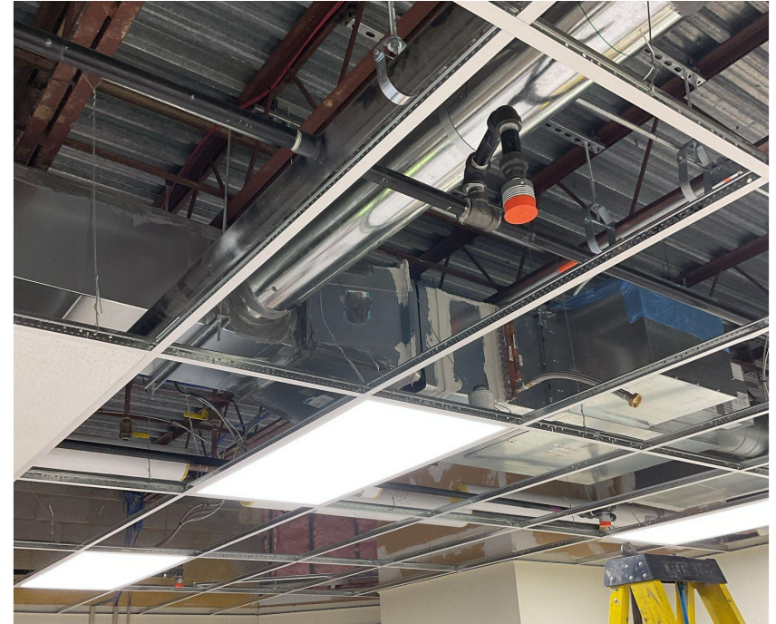
Variable Air Volume Terminal Unit
