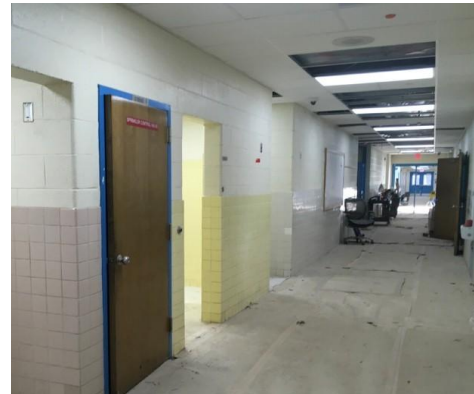
Corridor Ceiling Assembly and LED Lighting
