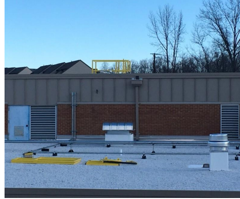
Roof Mounted Exhaust Fans, Gravity Vents, And Safety Rails
