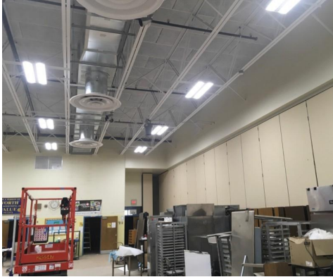
Cafeteria Air Distribution, LED Lighting and Sprinkler System
