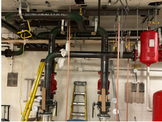
Hydronic Heating/Cooling Distribution Piping and Pump Stations
