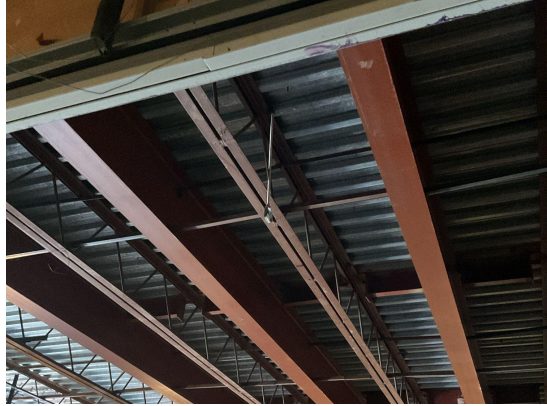
Structural Steel Supports for Roof Mounted Equipment
