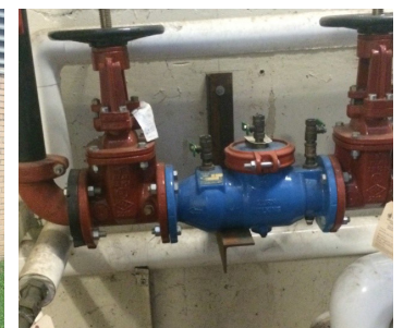
Sprinkler Supply Backflow Device
