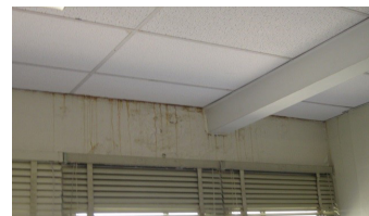
Water damage at building exterior wall.
