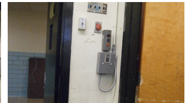
Typical Remote Control Cut-Off Station
