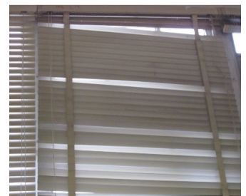
Damaged window blind
