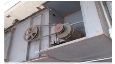
Existing H&V Unit Serving Gymnasium
