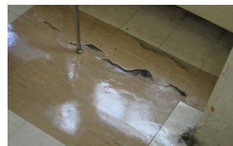
VAT with significant deterioration.
