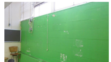
Water damage at building exterior wall.
