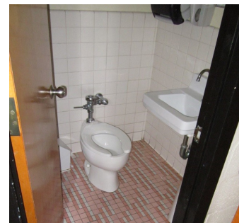
Bathrooms do not provide ADA clearances.
