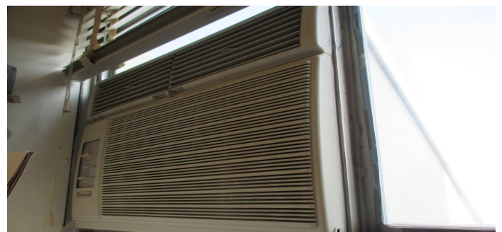
Typical Existing Window AC
