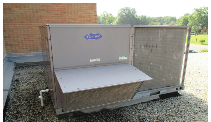
Existing Roof Top Units
