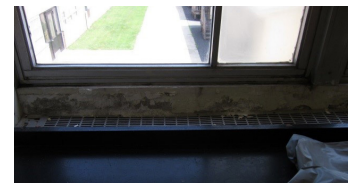
Water damage at window base.
