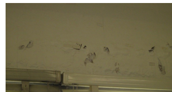
Deteriorating paint and plaster.
