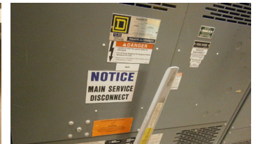
Main Service Disconnect Switch
