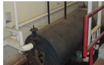
Existing Condensate Receiver/Condensate Pumps
