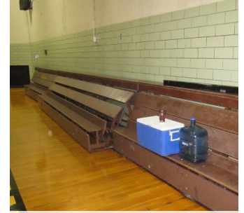
Current bleachers are due for replacement.
