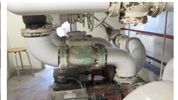
Existing Hot Water Pump
