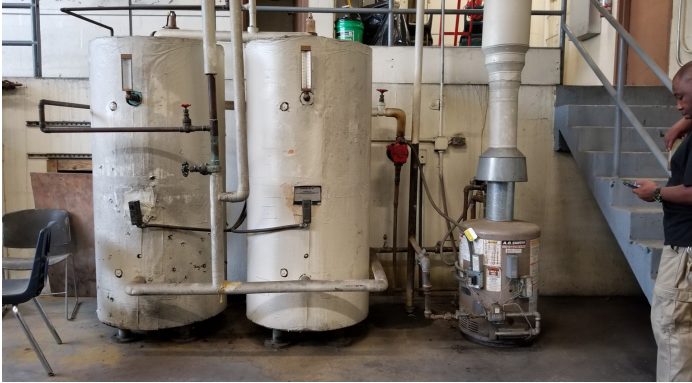
200 gallon hot water heaters
