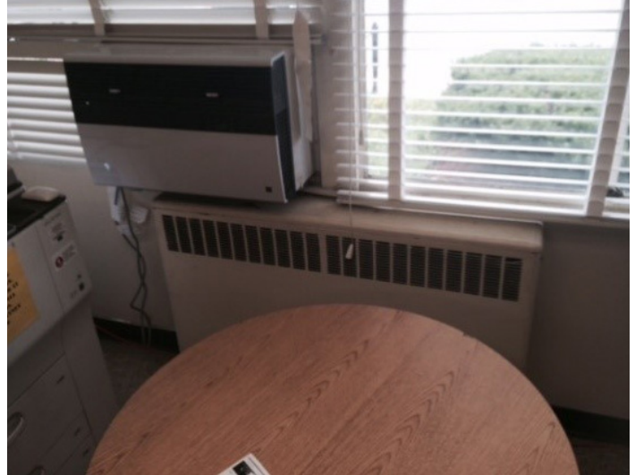
Typical classroom heating unit and window AC
