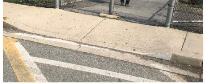
Existing sidewalk not ADA compliant
