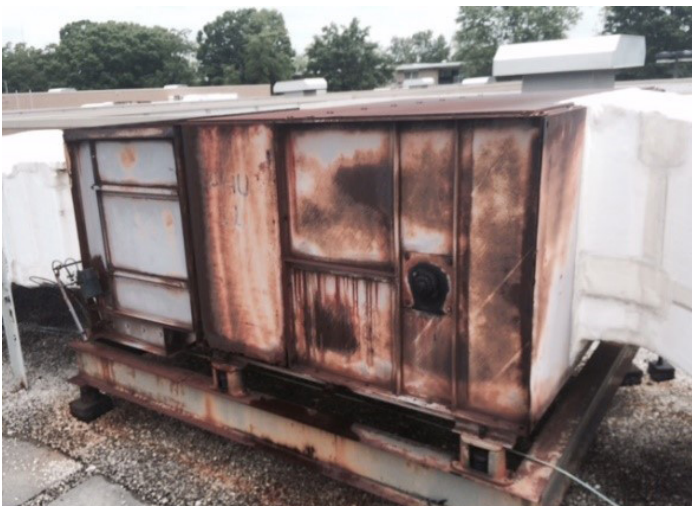
Rooftop Unit in Poor Condition
