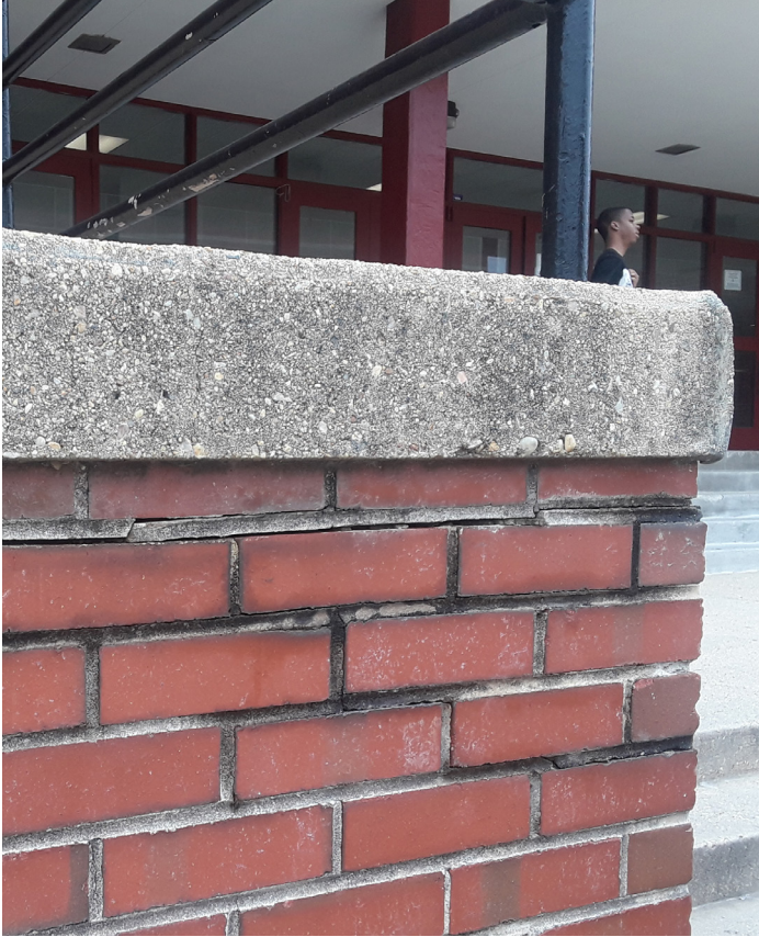
Grout damage at entry
