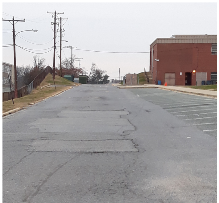
Patching at damaged asphalt
