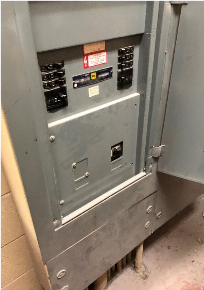
Typical surface mounted panel in workshop
