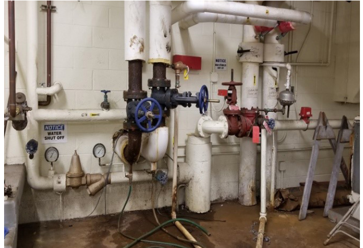
Incoming domestic water service
