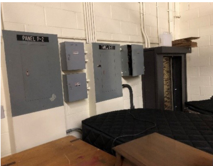
Typical panel boards
