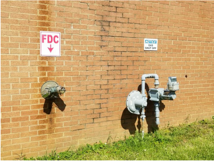
Gas service supply to boiler room
