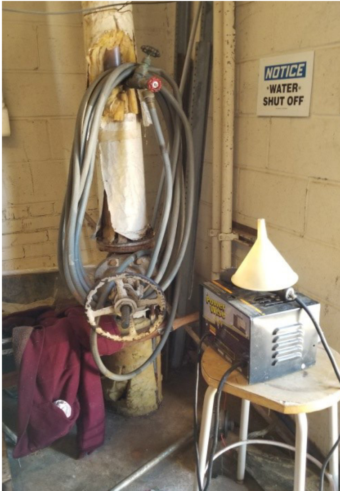
Domestic water & fire service in mechanical room
