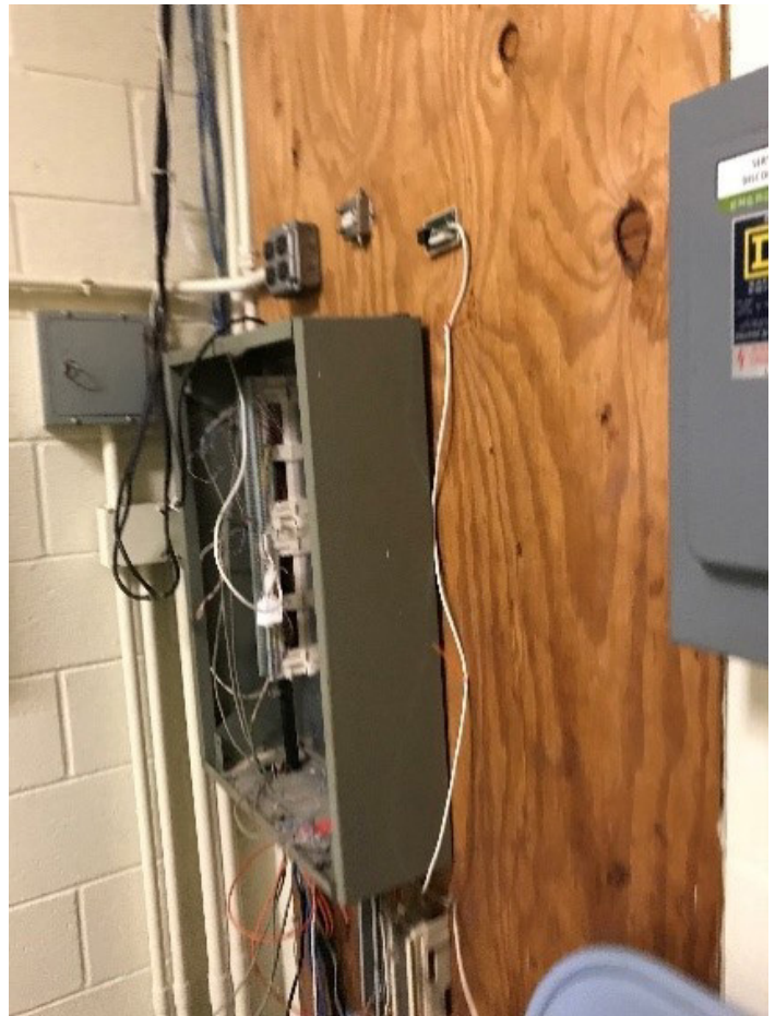
Data rack mounted in ticket office
