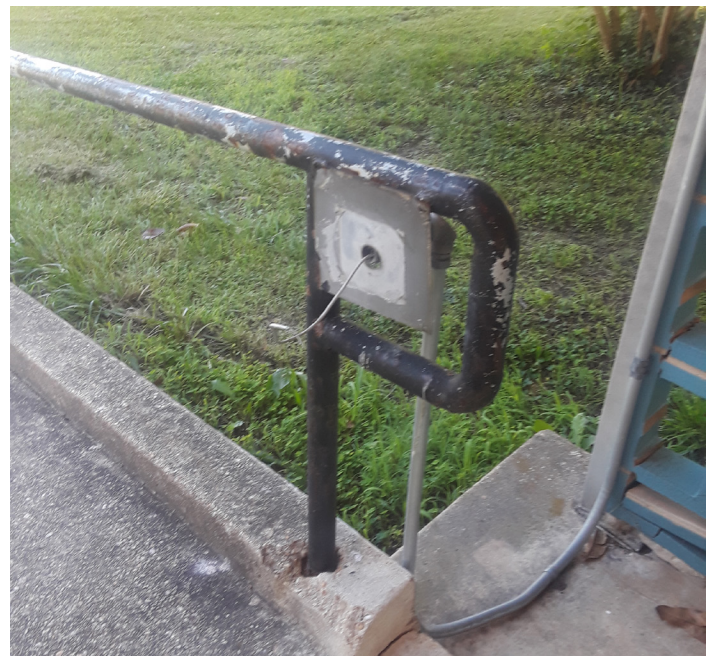
Ramp entry with missing push button
