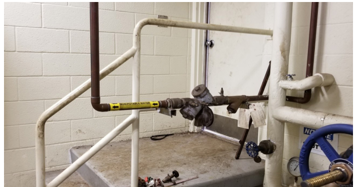
Mechanical makeup water line
