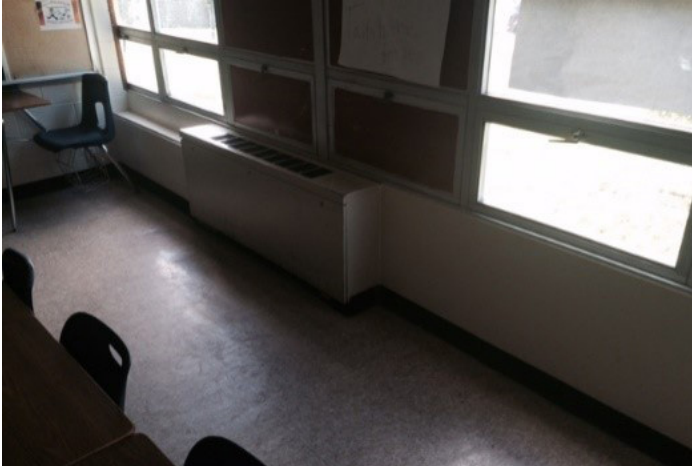
Typical classroom FCU
