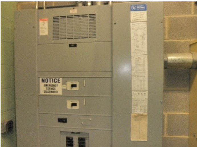
Emergency generator panel EMDP
