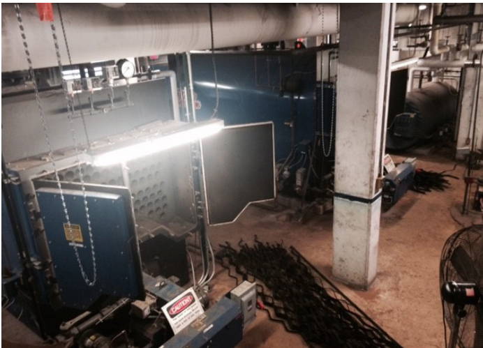
Firebox heating water boilers
