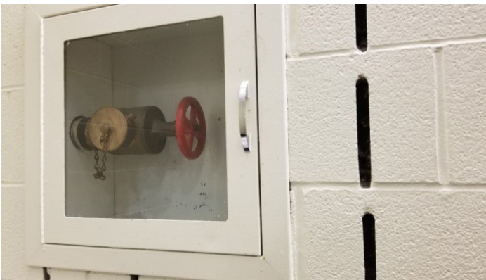
Fire hydrant next to stage
