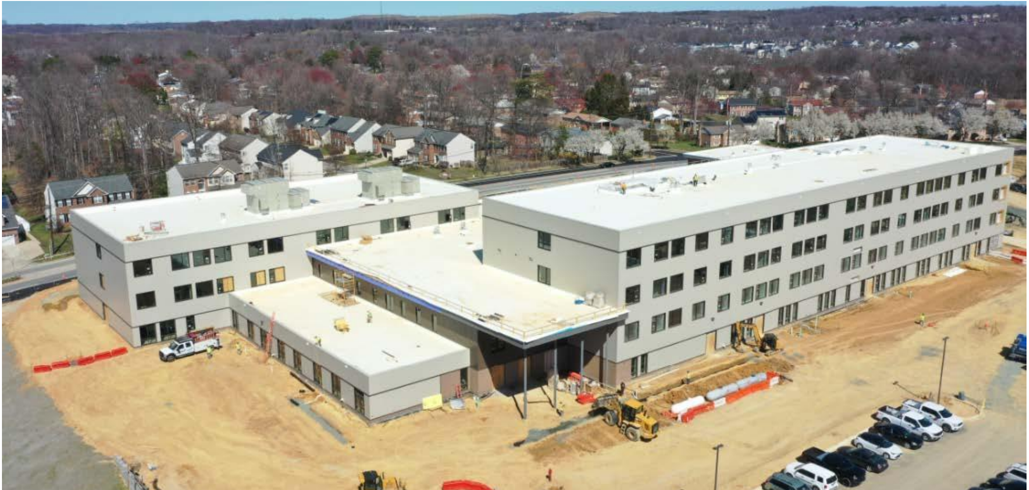
Aerial View of the West Entrance Side of the Building in Late March
