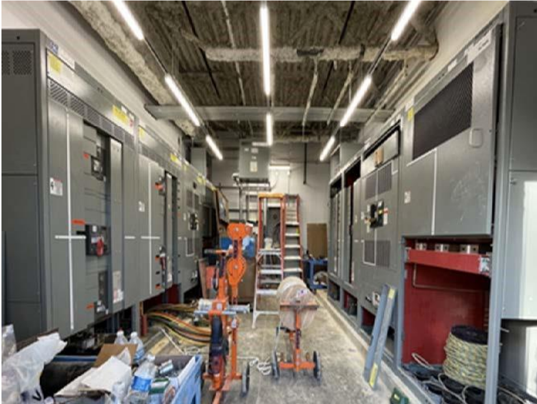
Main Electrical Room - Switchgear
